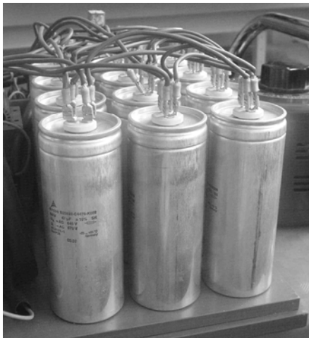
Fig 3c: discharging capacitor block
